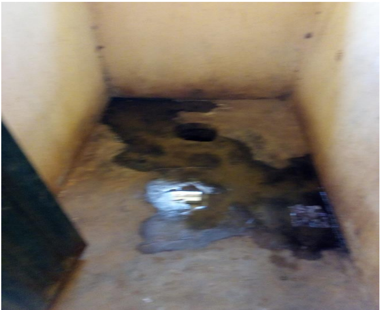
Plate 1 : Insanitary Pit toilet in the Study Area
