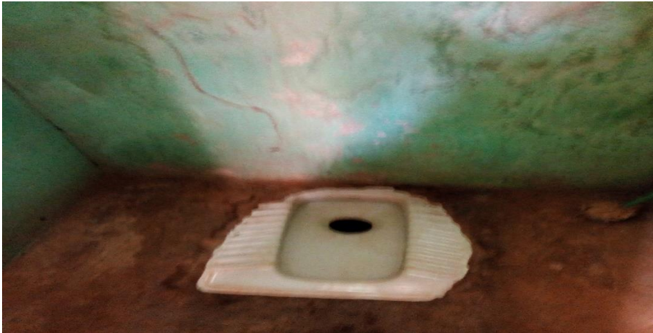
Plate 2 : Insanitary Water Closet toilet in the Study Area
