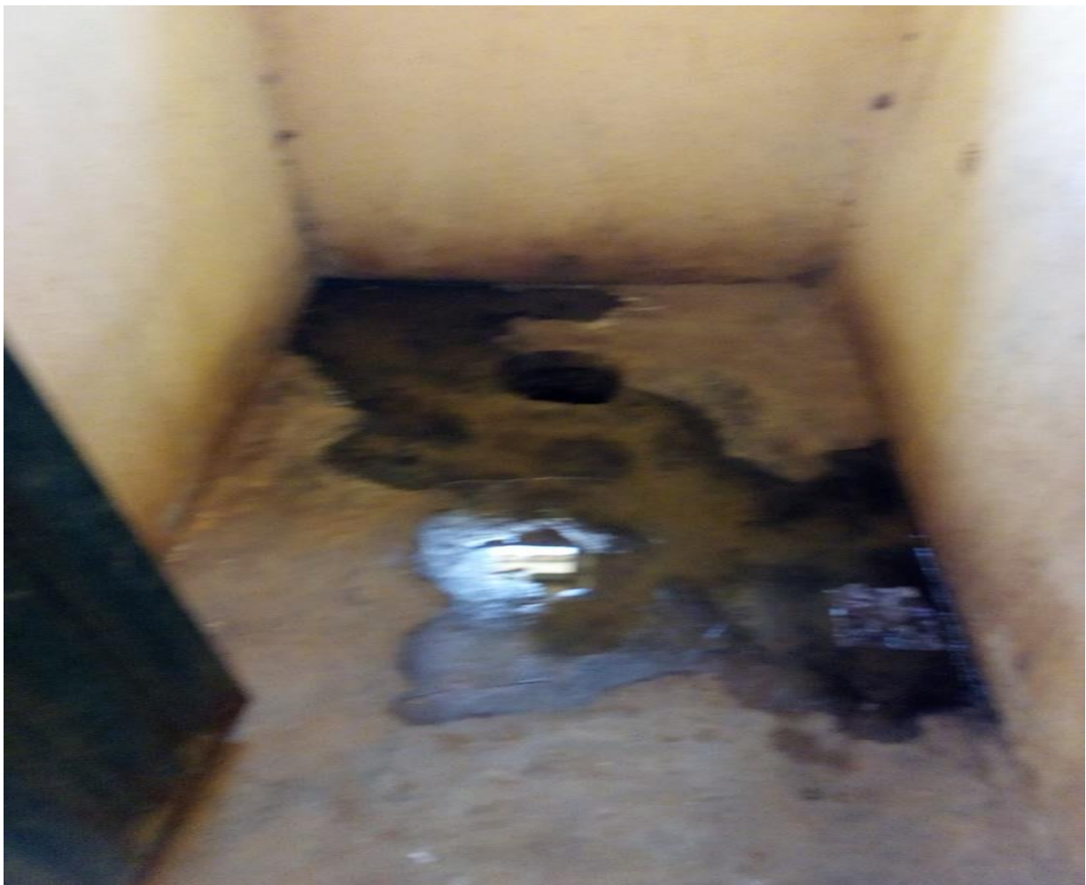
Plate 1 : Insanitary Pit toilet in the Study Area
